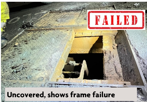
Patched following a frame collapse
