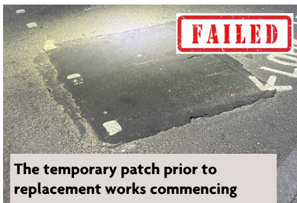
Uncovered, shows frame failure
